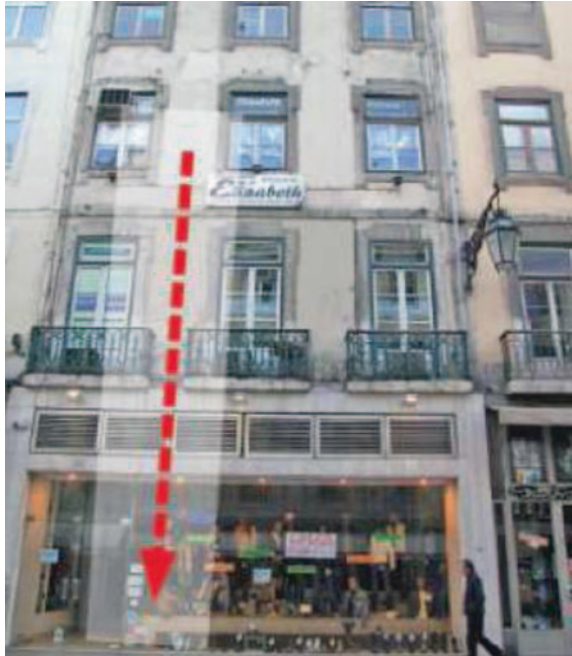
Fig. 22 Cut of columns at ground floor level [21]
