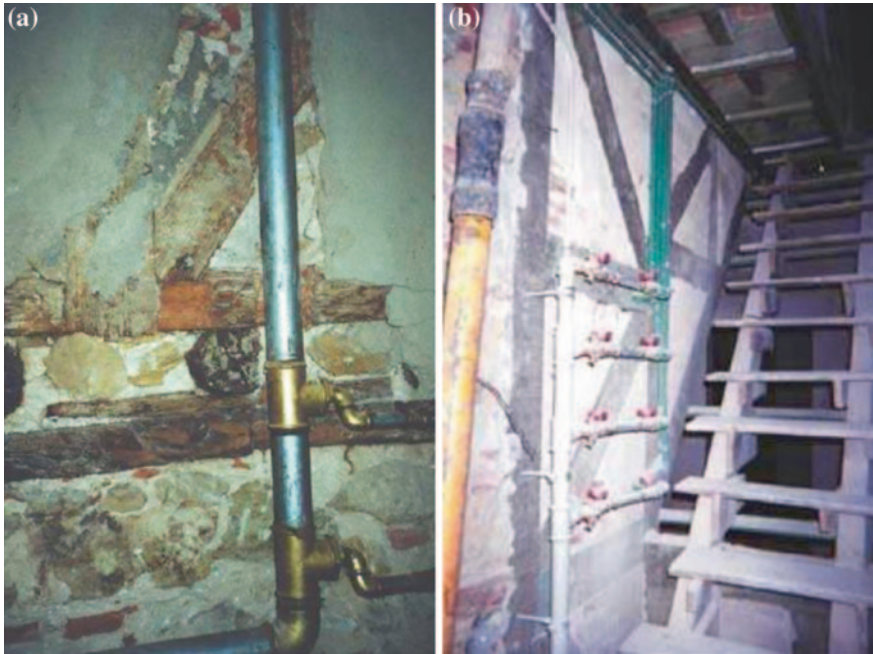
Fig. 20 a Cut in frontal wall to introduce pipes and b pipes crossing wall in the perpendicular direction [20]
