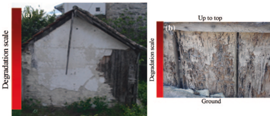
Fig. 12 Ground depending pathological effect. a Deteriorated façade. b Biological attack effect
