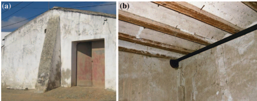
Fig. 8 Strengthening of rammed earth walls by means of: a buttressing [20]; b tie bars [5]
