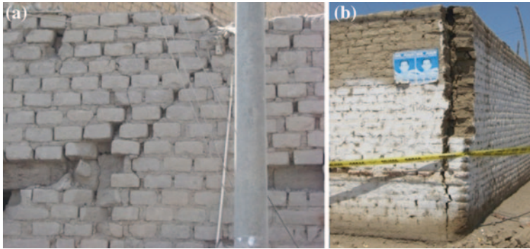
Fig. 20 Typical crack patterns in adobe masonry walls. a Stair crack shape (concentrated on mortar). b Vertical crack (fracture of bricks)
