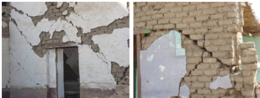
Fig. 9 Typical X-cracks on adobe walls due to in-plane actions
