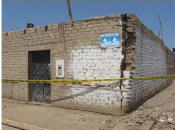
Fig. 7 Vertical crack at the corner of an adobe house, Pisco earthquake, Peru, 2007
